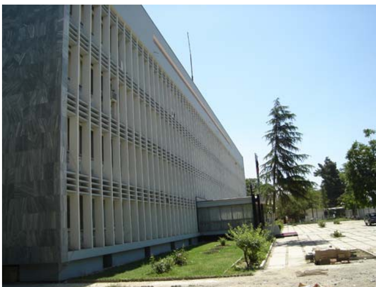
MARMARIN (OAA) Building repair works recently completed under Facility Domain of SCoG project – June 20, 2007
