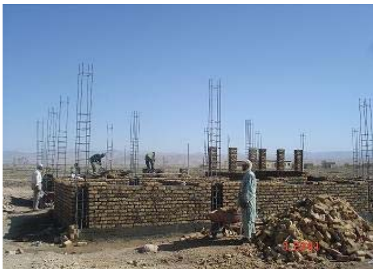
Construction of a health clinic in Pashtun Zarghun District as a result of DIAG compliance in Herat.
