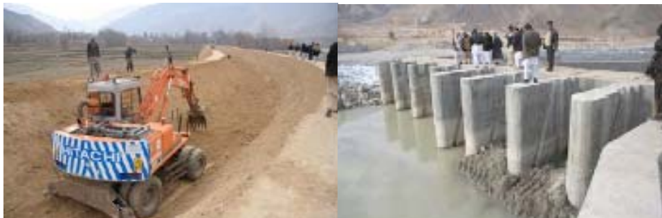
Left: Digging a 1.4 km canal to the MHP power house in Farkhar District
